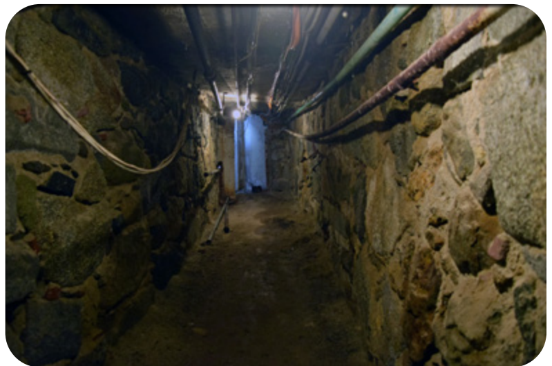
The tunnel from the Administration Building to the bowling alley under the Old Chapel on the Tewksbury Hospital campus.
